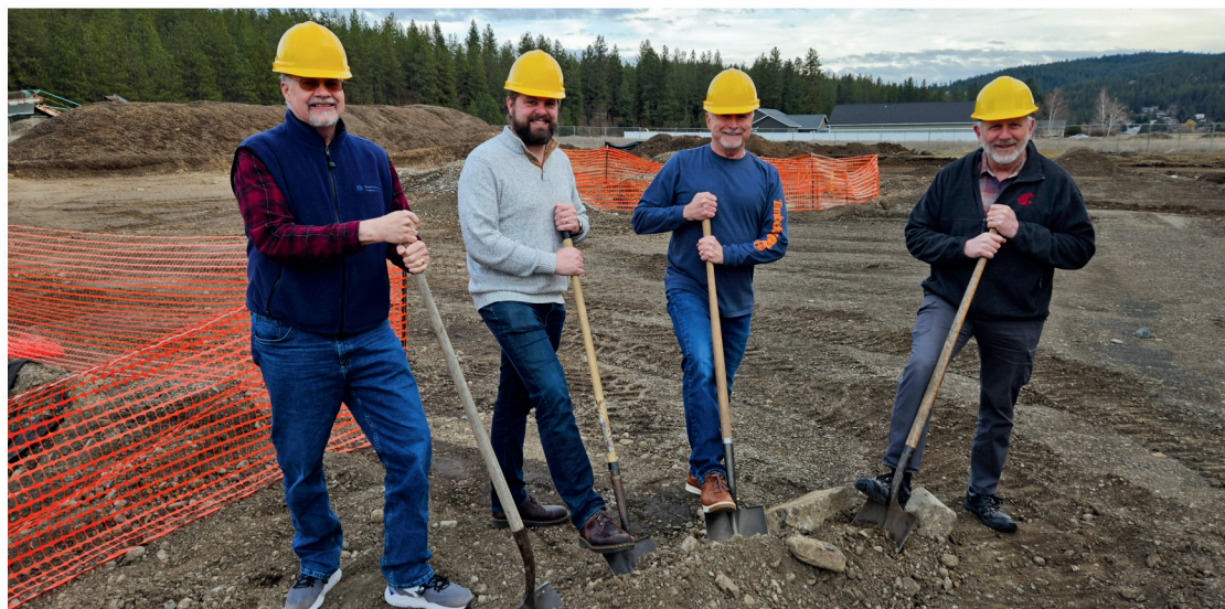
We have broken ground on Phase 1 of the Building Project! If you are interested in contributing financially to the project, pledge packets are available at the Welcome Counter. Pictured (from left): Gerry Caesar, Chris Martin, Ben Orchard, and Doug Snook.
